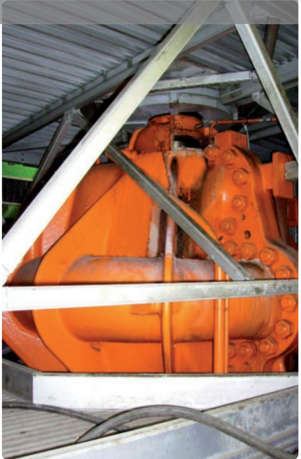
High-power pumping station for Syndicat des Eaux d'Ile-de-France.
