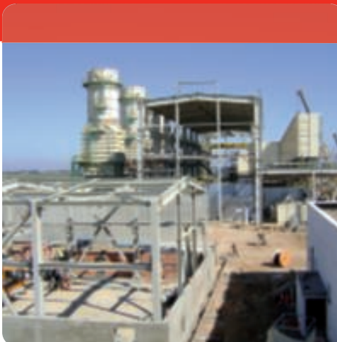
Relizane open-cycle power plant in Algeria.
