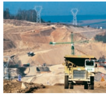
Earthworks on the LGV Est, the largest railway project currently under way in Europe (GTM Terrassement).
