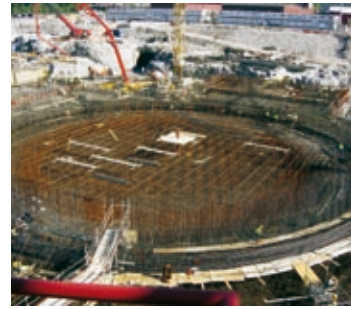
In Finland, Freyssinet is installing the prestressing for a new-generation EPR nuclear reactor.
