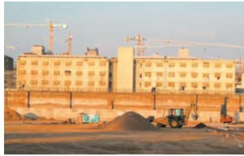
Construction of three prisons in Chile, as part of a public-private partnership which includes management of the sites for 20 years.
