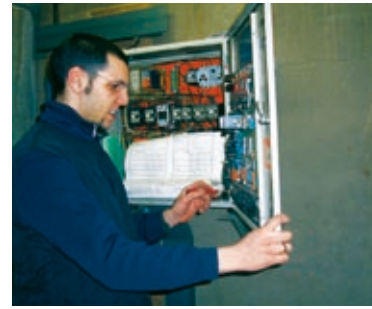
Sogea Construction, with its Manei brand, is a major player on the multi-technical and multi-service building maintenance market in the Paris region.
