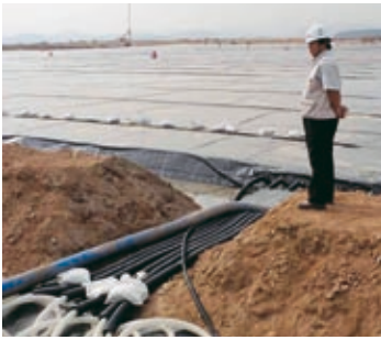
Consolidating a 295,000 sq. metre surface in the port of Kwang Yang, South Korea, using the Ménard Vacuum process.
