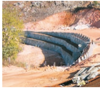
Mbabane bypass in Swaziland, where 36,000 sq. metres of Terre Armée reinforced earth were applied.
