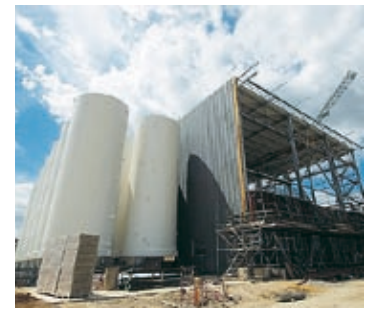
Sludge treatment unit for the Valenton purification plant in the Paris region (GTM Génie Civil et Services).
