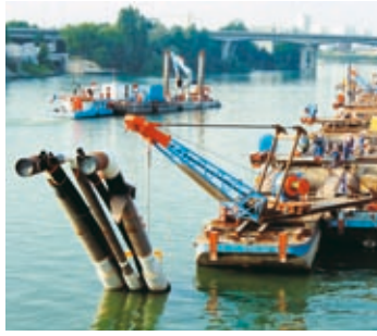
EMCC, a subsidiary specialising in marine and river works, laying natural gas pipelines under the Seine.
