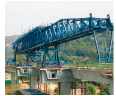
Heaving lifting operation on the Shenzhen Western Corridor Bridge in China, which Freyssinet is also equipping with cable stays and bridge bearings.
