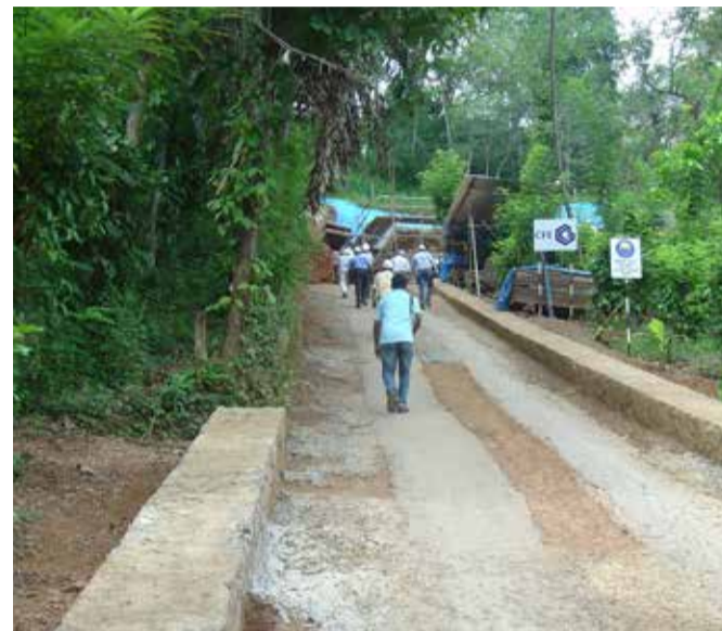
▲ Construction of a drinking water station in the mountains - Kolonna (Sri Lanka)
