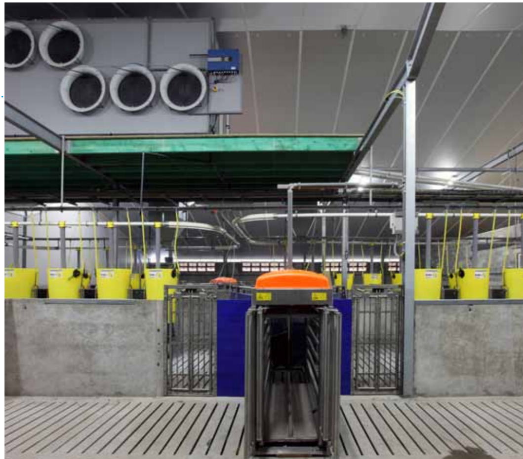
Electromechanical installation in the agriculture industry – Wuustwezel (BE)
