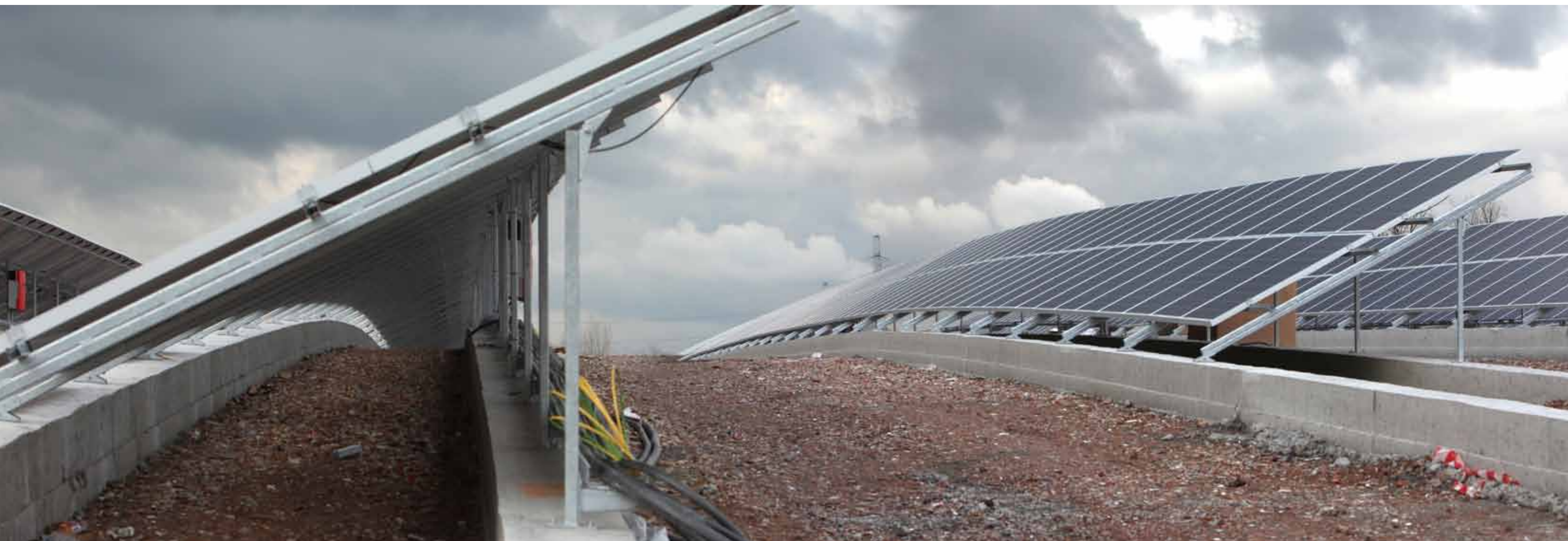
Development and construction of one of Belgium's largest solar power farms at Lier (BE)
