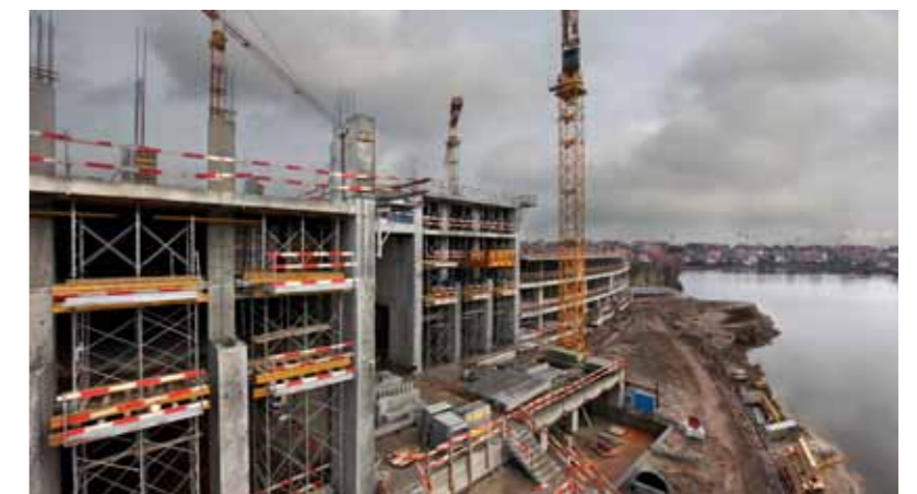
Construction of apartments and a hotel for the 'La Réserve' project - Knokke (BE)
