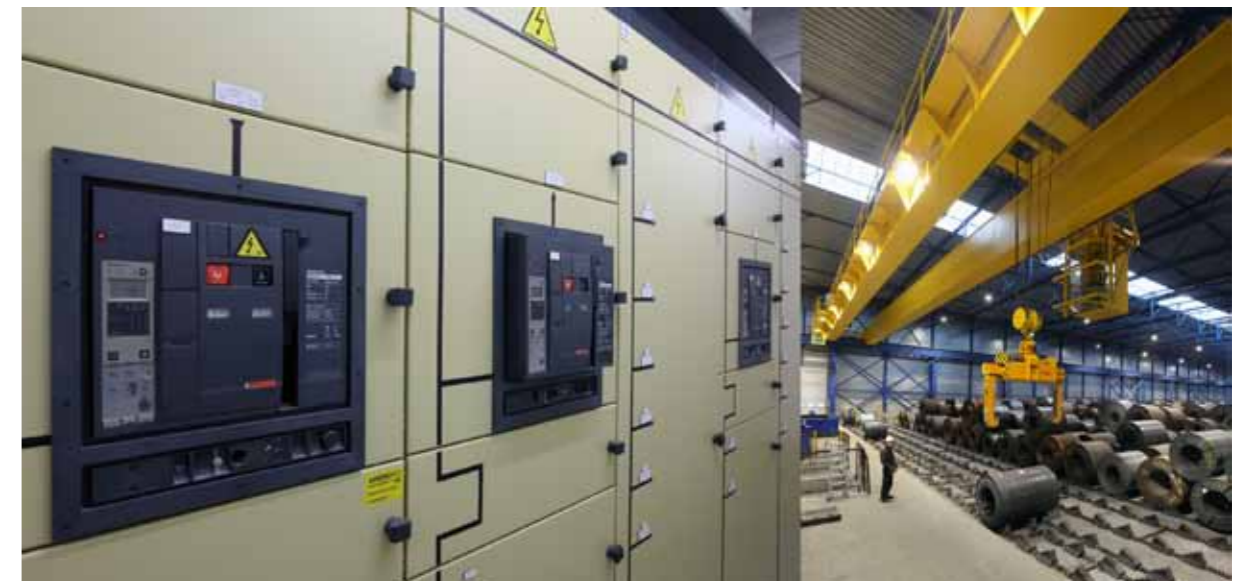
Study and execution of electrotechnical works in a production hall and office building for LSC – Bree (BE)
