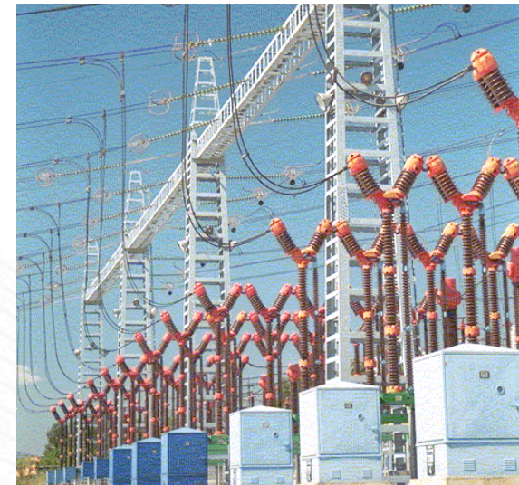
Transformer stations (ENDESA)
