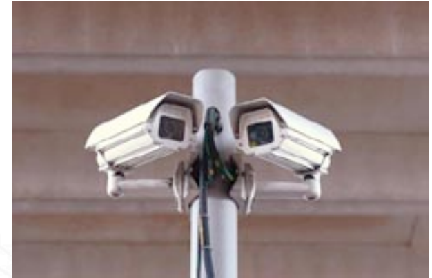
Video surveillance (low voltage)
