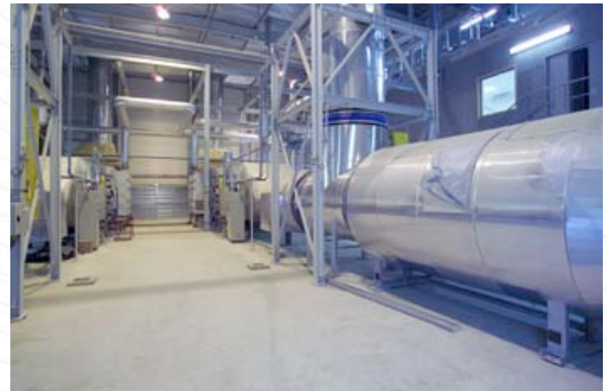
Climate control (A380 hangars – Toulouse)
