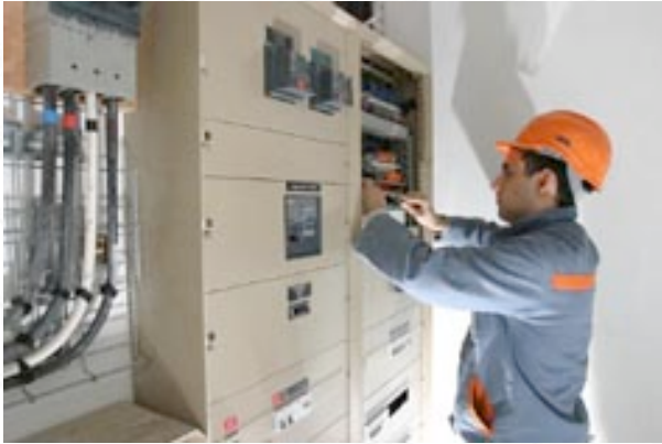
Power supply (high voltage)
