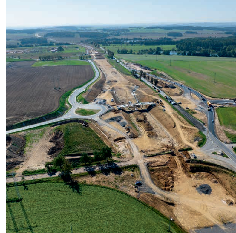
↑ Work on the D4 motorway, the first being built under a public-private partnership in the Czech Republic.
